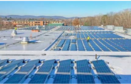
City of Keene DPW-Police Building, Wastewater Plant 2 MW (2018)
