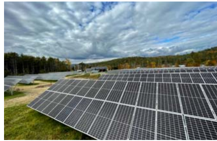
Town of Hanover Water Department, WWTF, Town Roofs 2 MW (2016-21)
