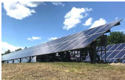
City of Lebanon Wastewater Plant + Town Roofs 836 kW (2019)
